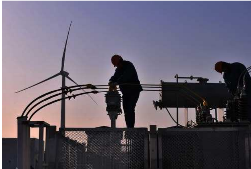
Workers building a wind farm for China Longyuan Power Group Corp in Chuzhou, Anhui province. The company has bought rights to develop a wind project in Canada. [Photo/China Daily]
