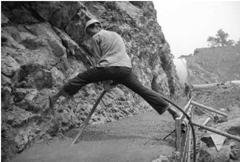
Workers at the construction site of a highway tunnel in Chaohu, Anhui province, in June. The authorities are aiming to expand the nation's transport network in the coming year. [China Daily]
